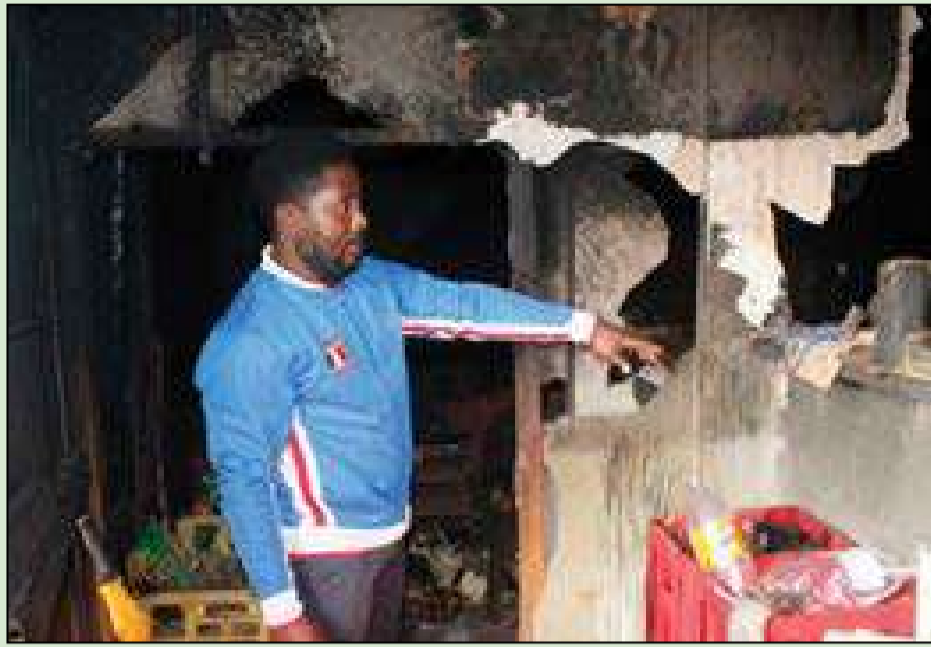
Vhulenda Nemanane points to the damage, caused by a fire at his shop in Khubvi village last week. Photo: Victor Mukwevho.
